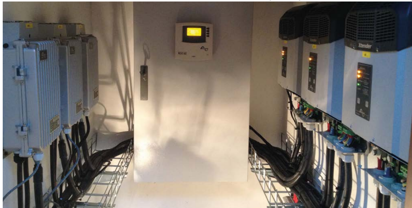
Self-consumption system for industrial building
